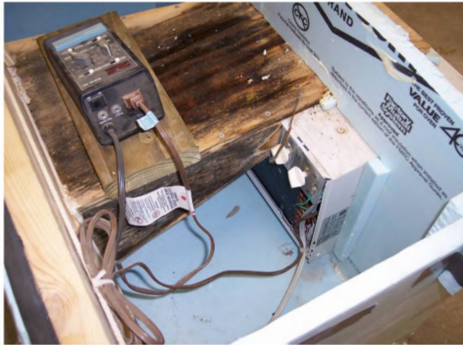
Figure 3-3: Insulated Box Surrounding the A/C Unit
